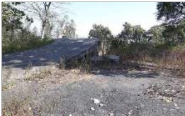
Before- Unsecured mine entry
