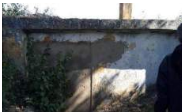
Before- Open and Unsafe Entry Point
