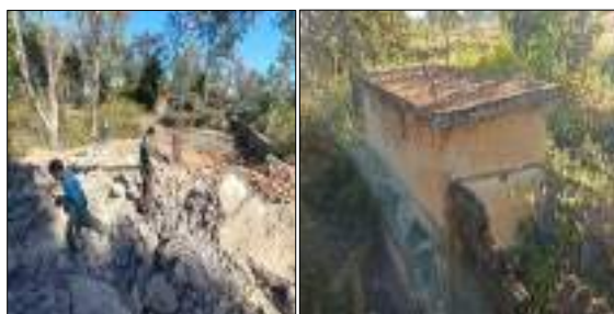
Before- Debris and Remnants of Existing Structures
