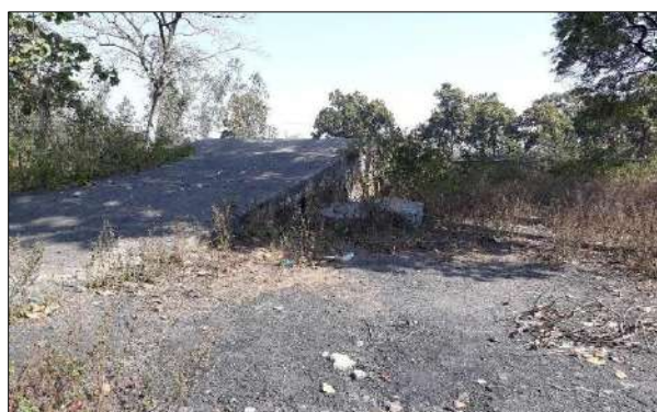
Before- Unsecured mine entry
