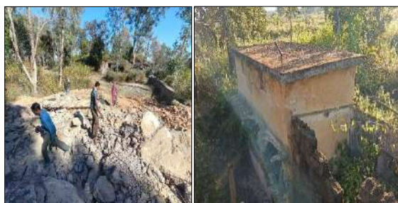
Before- Debris and Remnants of Existing Structures
