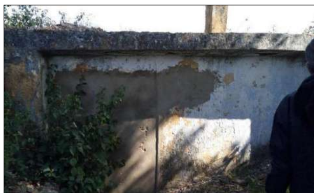
Before- Open and Unsafe Entry Point
